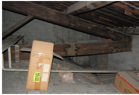
Figure 6 - Santa Chiara, Florence: Roof beams visible above the baroque vault. Photograph: Donal Cooper
