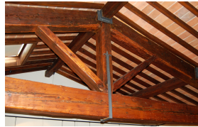
Figure 7 - Santa Chiara, Florence: Roof beams in the former nuns' choir. Photograph: Donal Cooper
