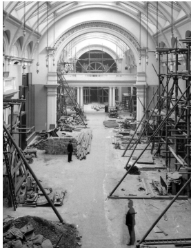
Figure 15. Gallery 50 under construction, late 1908 or early 1909. Courtesy of the Victoria and Albert Museum, London
