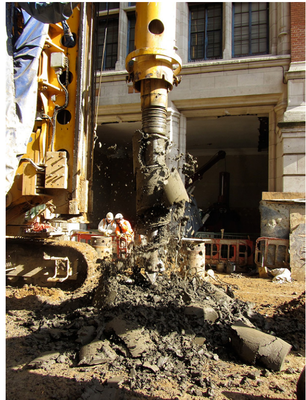
Figure 6 – Piling rig drawing clay out of the ground on the Exhibition Road building site. © Victoria and Albert Museum, London
